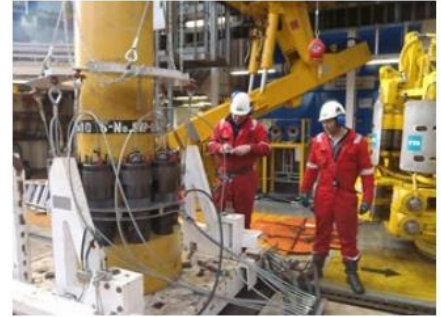
A WellPartner HP-Riser flange about to be made-up with special tooling on the drill floor of a NCS jack-up rig.
